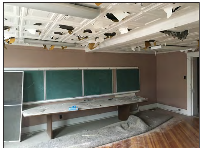
The second and third floors will need to be renovated before they can be occupied by SCCC.
